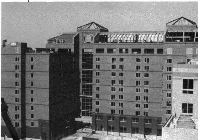
Construction began in 1989 on the Virginia Square complex in Arlington, Virginia, which will be used for FDIC offices, classrooms and a residential center for personnel attending sessions.
